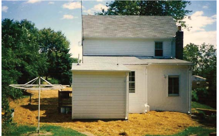
FHC installed a functional sewer system and drainfield and made other repairs to the home
