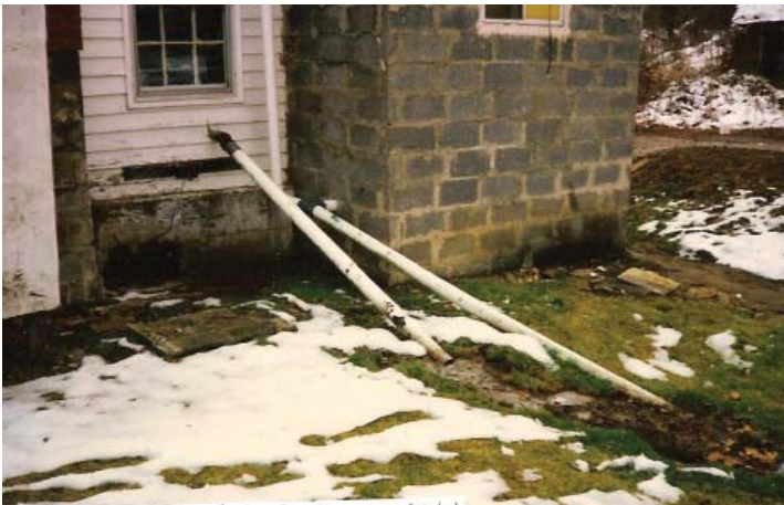
This pipe, leading out to the backyard was the sewer system for this home's elderly resident
